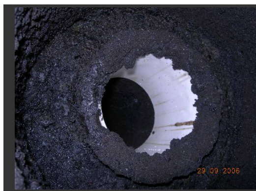
Fig. 2. Carbon steel vessel collects foulant; FPC liner (white) prevents fouling
